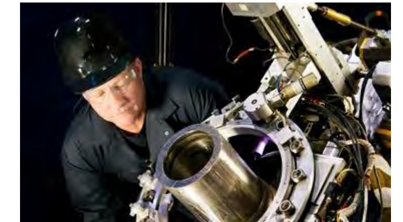
Pipe and Piping Services
