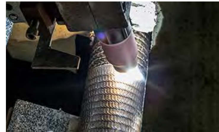
Heater and Furnace Services
