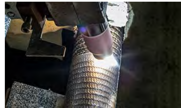
Heater and Furnace Services
